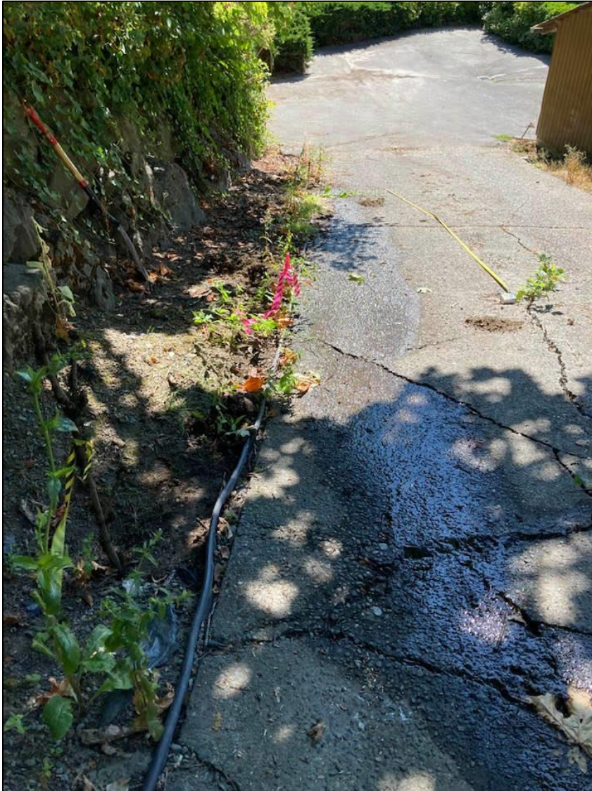
Photo 7. Seeps draining out of lower driveway adjacent to Wetland A (photo taken 7/23/21).
